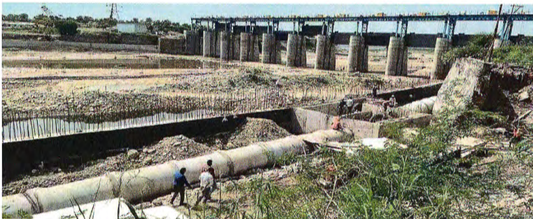
Picture showing Interceptor Drain On Right Bank
